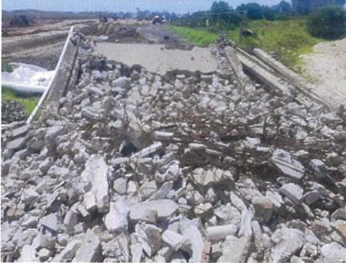
Photograph 4: ACM impacted bridge rubble prior to removal.
